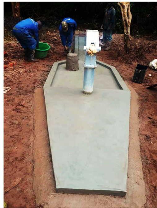
Community members putting the finishing touches on a cement apron slab, which protects the groundwater below the waterpoint (Credit: WW/Walter Chinangwa, 2020)
