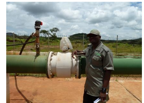
New protocols for monitoring water use and abstraction will drive efficiencies and compliance
